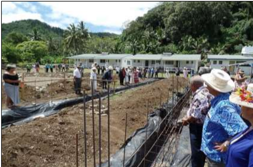
Laying of foundation, Takamoā multi-complex hall, looking eastward. Student quarters in background.
