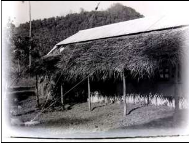
Kikau verandah being constructed to shade the west side of the station
